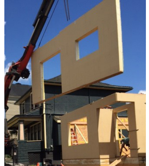
Image 1: Installation of a prefabricated wall assembly for a high performance new home under construction in New Westminster next to a protected heritage building.
