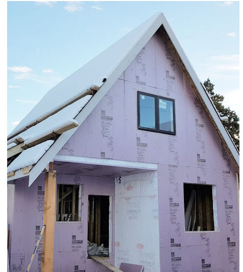
Image 1: A Single Detached Home designed to meet Step 4 of the Step Code, with exterior insulation shown during construction.
