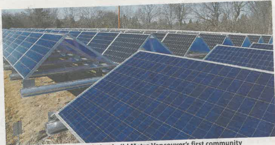
New Westminster has decided to build Metro Vancouver's first community municipal solar array — dubbed its Urban Solar Garden. — THE ASSOCIATED PRESS FILES
